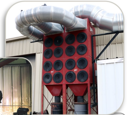
Source Capture Arms ducted to central system located outdoors returns clean, heated/cooled air to facility.
